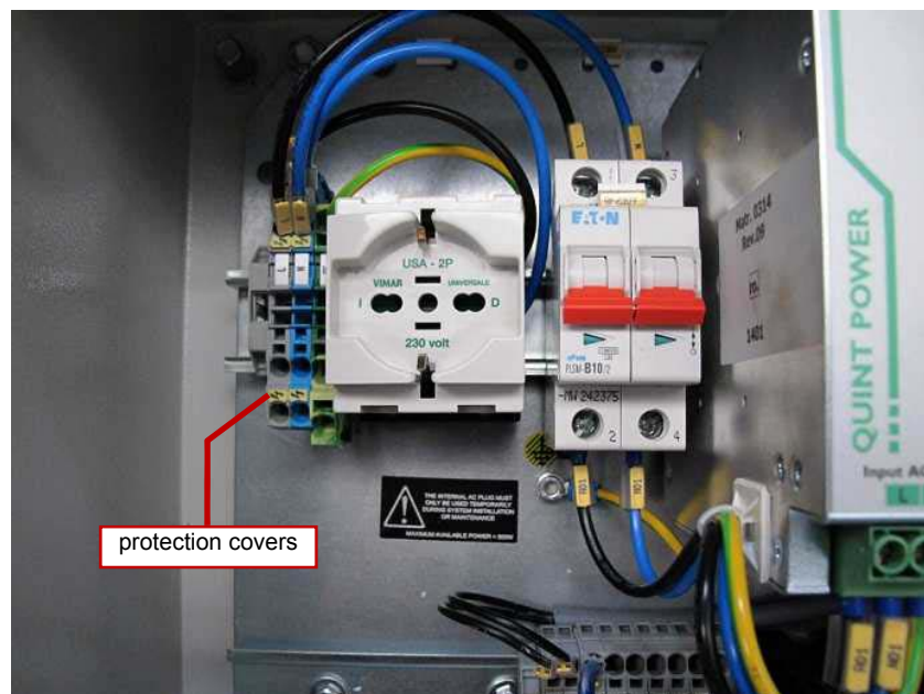
Figure 6 – PWR-480B AC Line Terminal Block with Protection Covers
